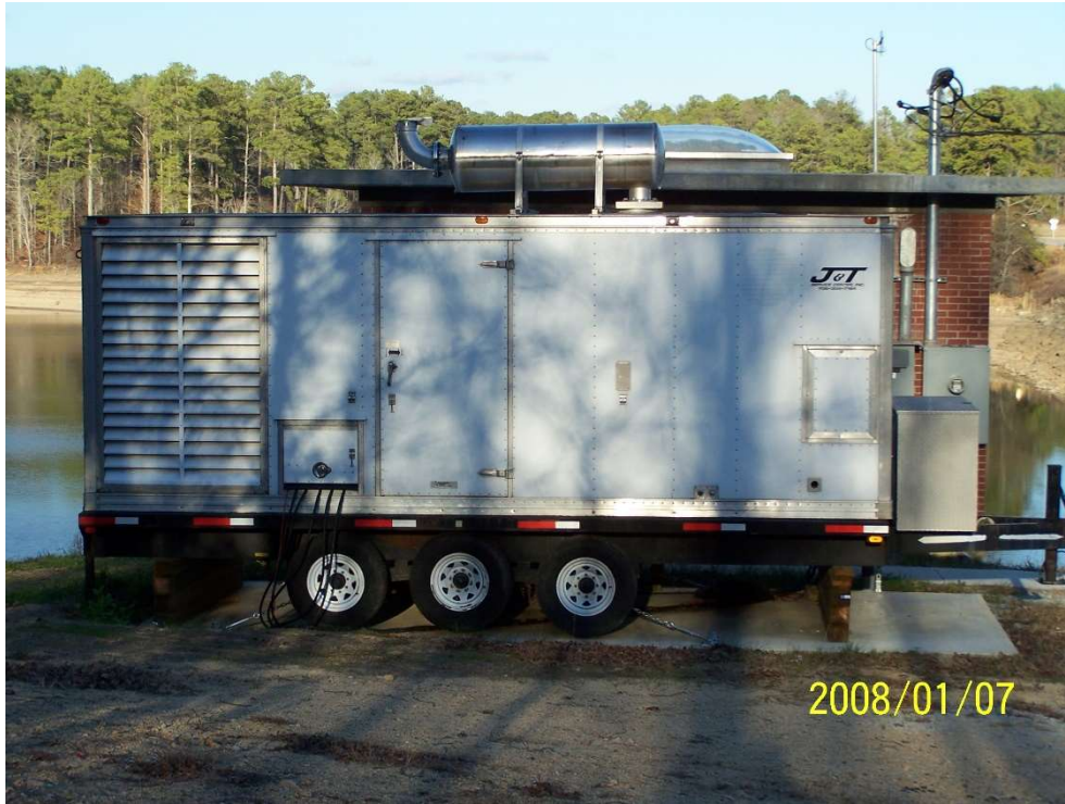
Emergency generator located at the Raw Water Station.
