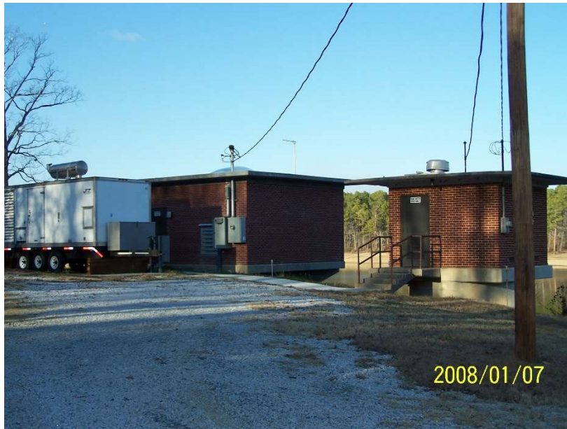
Left: The 2 million gallons per day Raw Water Station with backup generator
