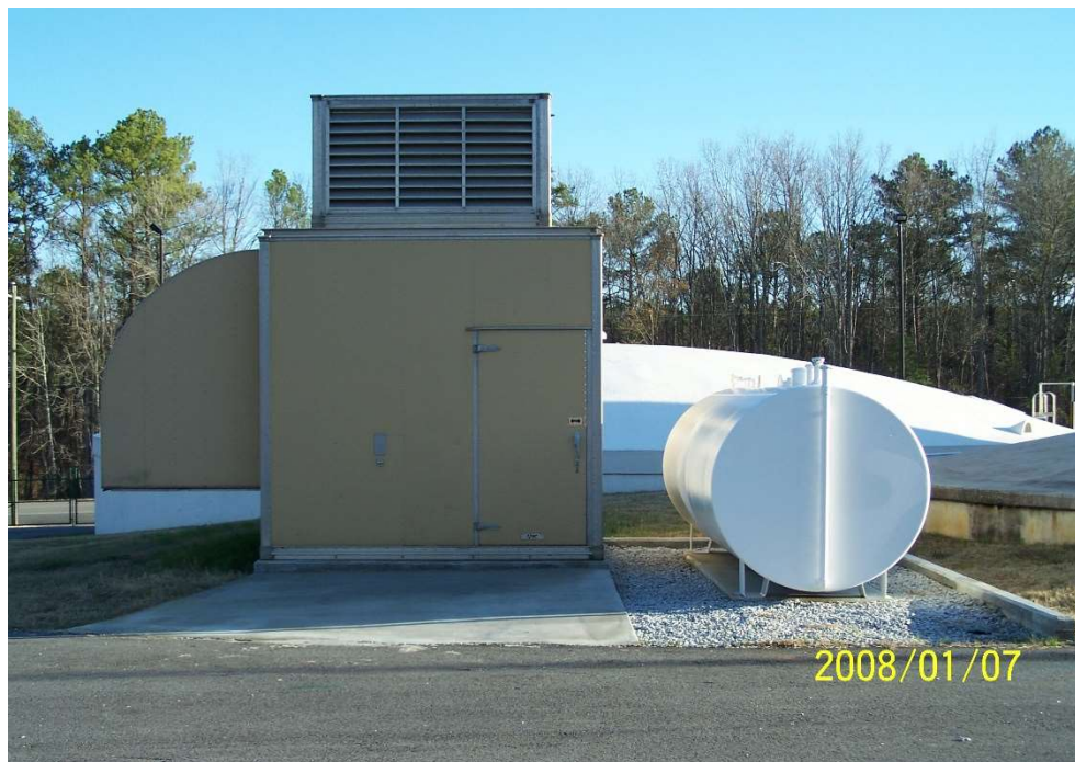
Emergency generator located at the James Allen Reed Water Treatment Plant
