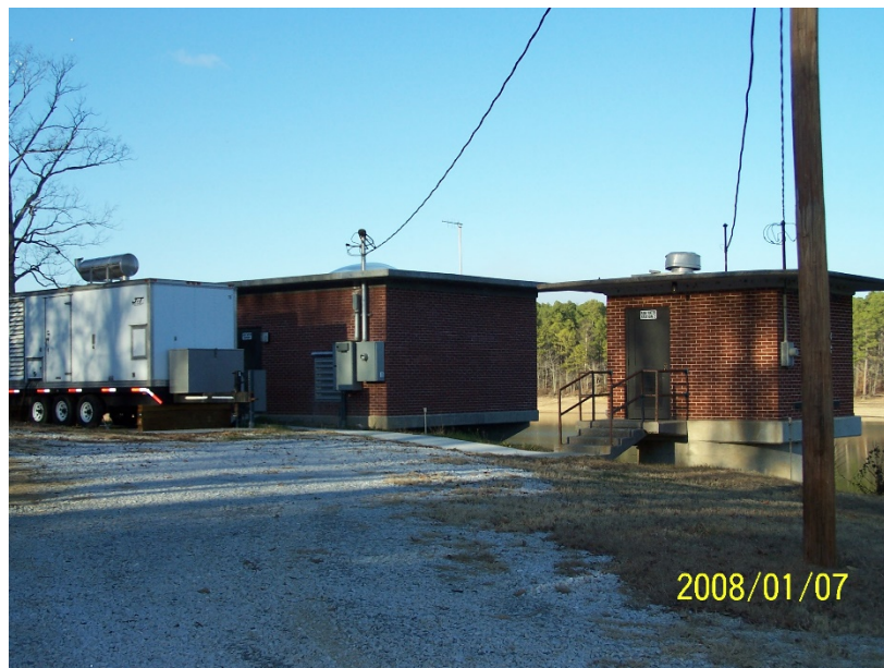
Left: The 2 million gallons per day Raw Water Station.
